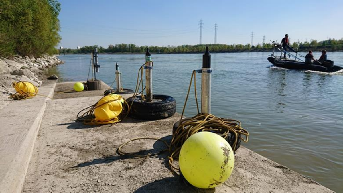
Figure 14: Hydrophones to be deployed as a receiver array ready for setup on the shore below the Freudenau hydropower station (© IHG/BOKU).
