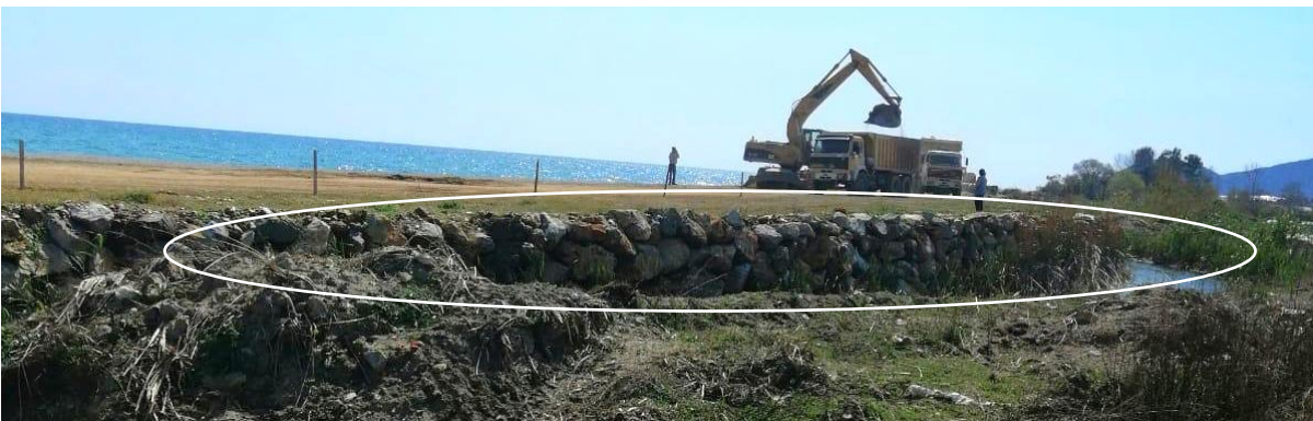
Fig. 4 | Karaağaç 31 March 2021: No restoration works have occurred for Sarisu Creek- the stone wall still remains. Heavy machinery removing the soil from the back of the beach in the background.
