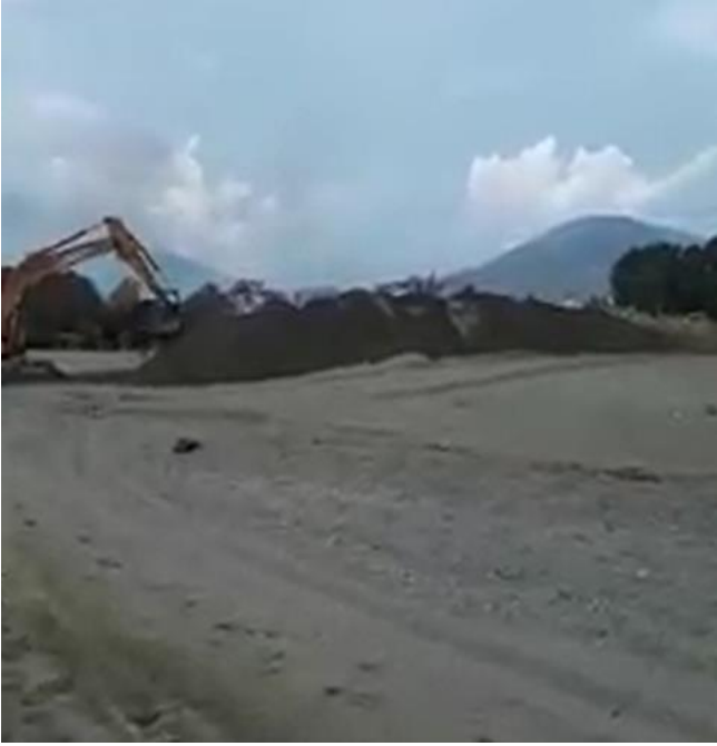
Figure 51 - The Municipality is Extracting Sand from the Beach – 1.11.2019. The Anamur Municipality applied to request permission from Anamur District Governorate for evacuation canal cleaning on 31.10.2019. However, they extracted trucks full of sand from the beach in contrary to the letter of permission. In addition, the Anamur District Governorate or any other authority did not make a complaint about this situation. See section 3.1 for full video and [R19] for more photos.
