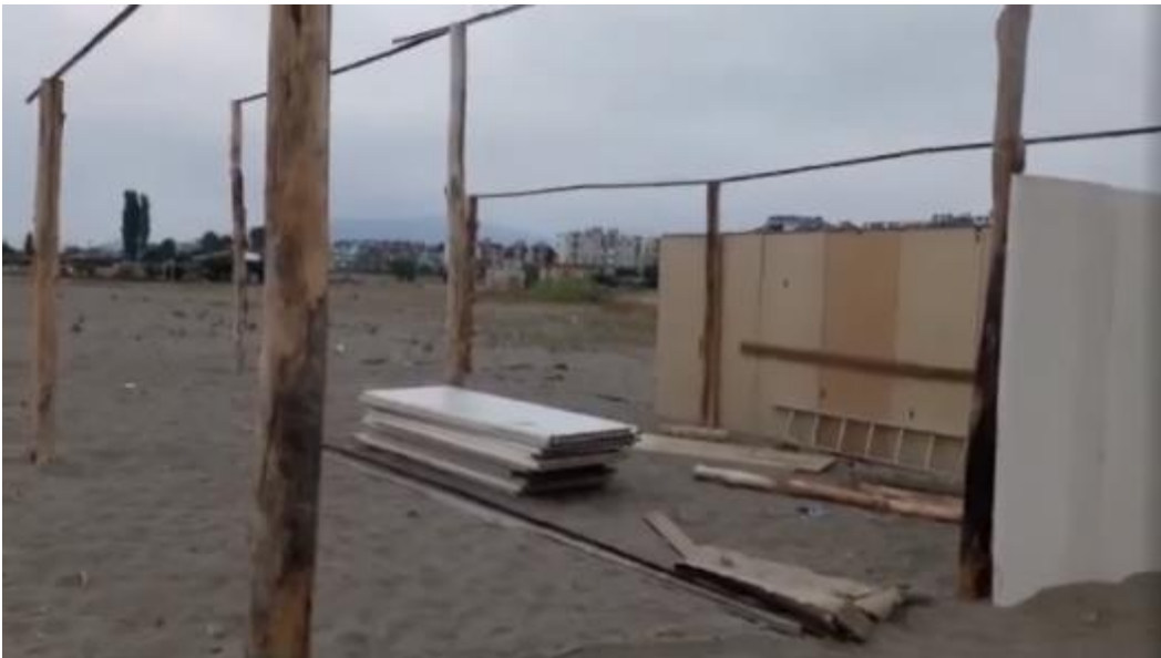
Figure 50 - Illegal Construction at Anamur Beach for a Water sports Company [R17]. Last year (2019), construction started on the beach by a water sports company, about 10 m from the shoreline. Initially, the authorities allowed the company to start the building. However, when people protest against it, the building was removed. Continual construction attempts show that authorities are not paying enough attention for protecting the sea turtle nesting areas.
