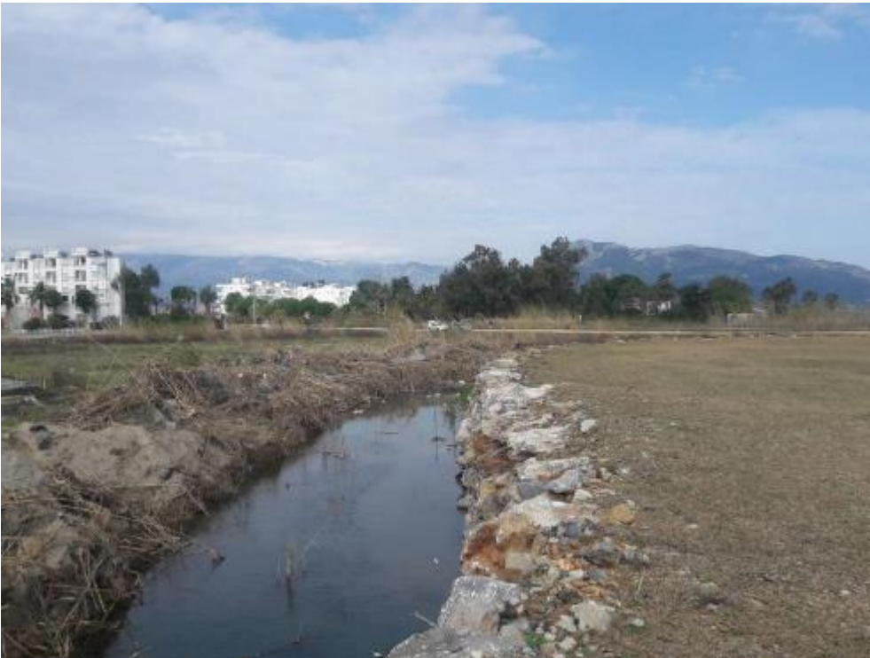
Figure 19 - Creek Construction - Reeds at both sides of the creek (as shown in Figure 7) are destroyed, a stone wall has been built along one bank of the Creek to prevent additional soil seeping into the Creek
