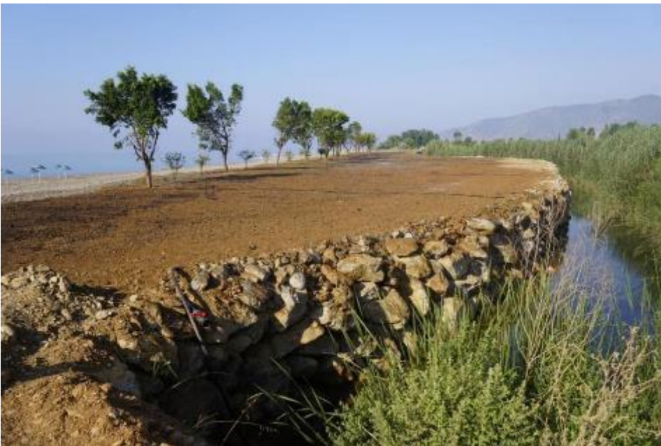
Figure 21 - Destroyed Reeds and Stone Wall Inside the Creek
