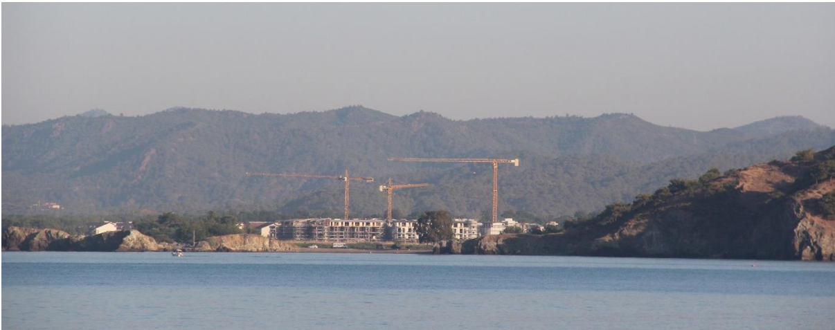
Fig. 5b. Fethiye SPA, Karataş. Construction site behind the small beach in Karataş, as seen from the Çalış beach.
