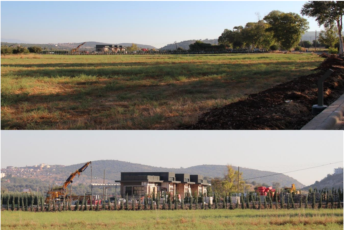
Fig. 4-5. Construction of the “visitor welcoming centre” with a large parking lot in front of it. The gendarmerie guard post is located right by the construction area’s entrance.
