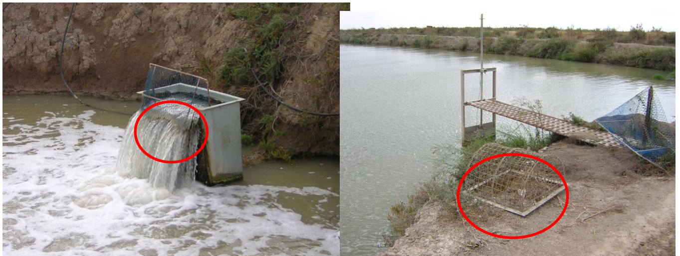
Figure 5.5: Inflow floodgate at the entrance of a semi-intensive unit equipped with a spherical filtering screen (red circle) mounted (left) and detached (right)
