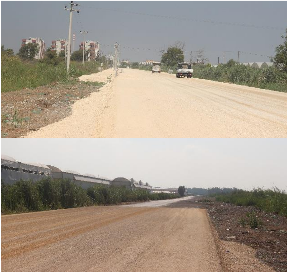
Fig. 39. Kazanlı, Section K1. July 2021. Construction work for broadening of the road behind the nesting beach.
