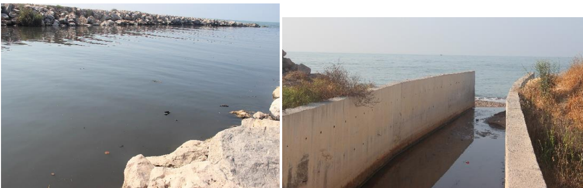
Fig. 46. Kazanlı. July 2021. Example of drainage channels reaching the sea Left: K1 southern end. Right: K2-K3 border.
