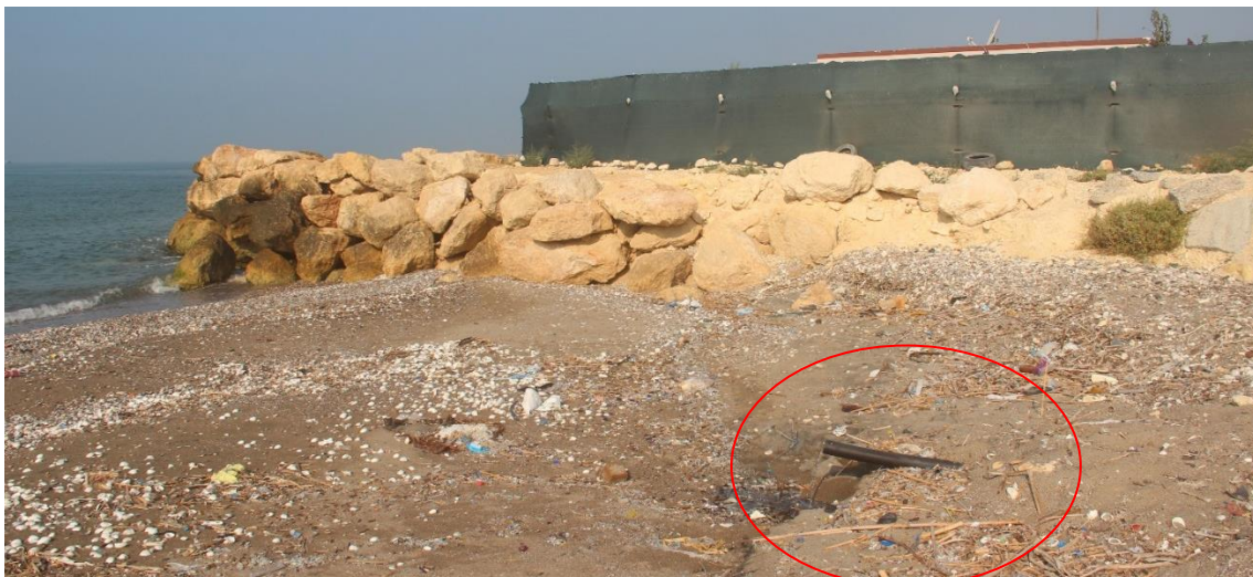
Fig. 10. Kazanlı. Section K3. July 2021. Small drainage pipe at the section's northern end.
