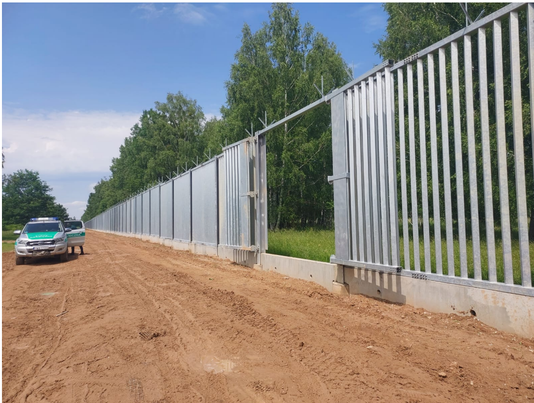
Photo 2. The appearance of the dam on the Polish side of the border with a crossing for large animals and culverts for small animals.
