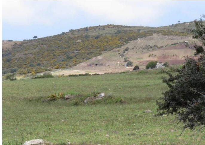
Heavy earthworks, vegetation removals and renovation of “stidia” (traditional stony sheep/goat corral) near Lara MPA.
