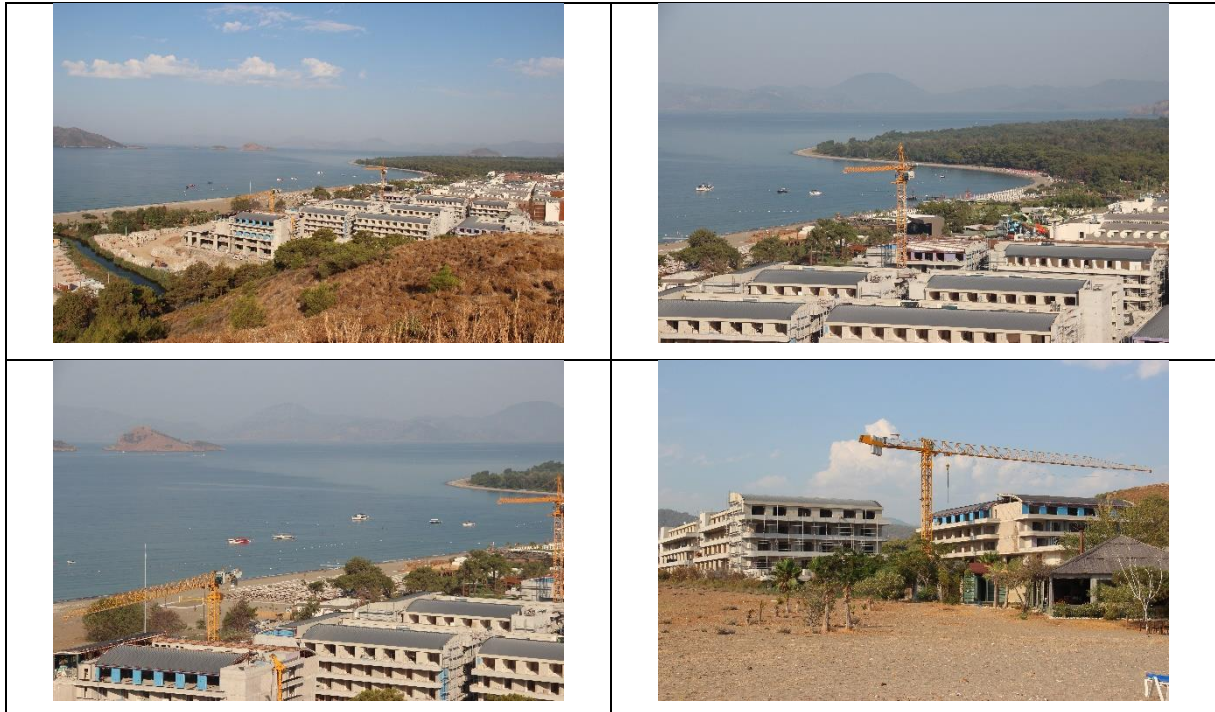
Fig.8. Fethiye SPA, Yanıklar. Construction of the new hotel almost finished. Note the boats, the cranes, the enlarged beach usage area of Liberty Fabay invading the nesting zone in 8c, and the artificially planted trees of Deniz İncisi in 8d.
