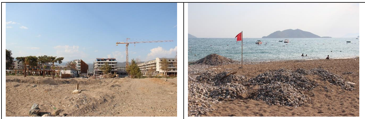
Fig.39. Fethiye SPA, Yanıklar. Sand extraction in front of the new hotel construction (Liberty).
