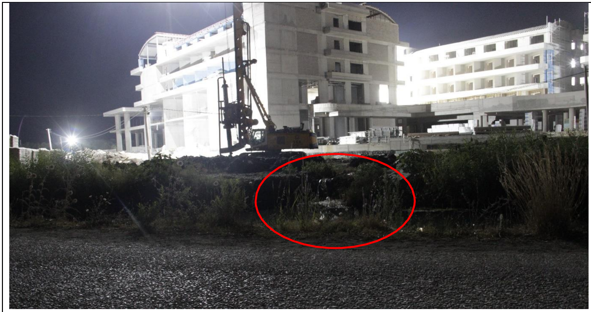
Fig.62. Fethiye SPA, Yanıklar. A pipe draining directly into the channel bordering the construction site of the new hotel of Liberty Group, further contributing to habitat damage.
