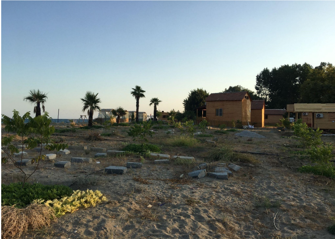
(Fig. 6o) Basement preparation is going on for additional bungalow houses to be built on the beach
