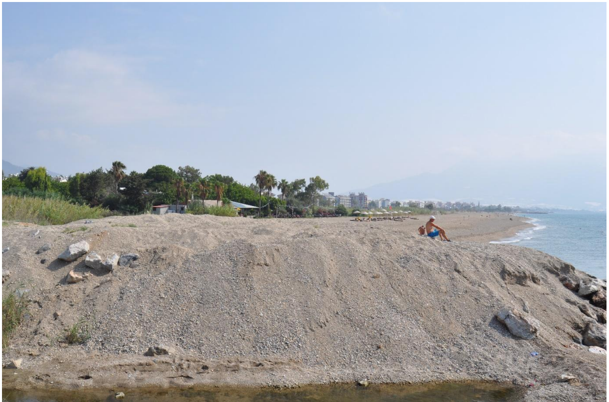
(Fig. 3b) Sand extracted from canal (Fig. 3a) was relocated to these piles, during the activities carried out within the scope of the beach arrangement project.
