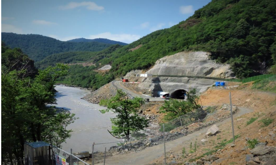
Lower Namakhvani dam and tunnel construction site, July 2021. Credit: Andrey Ralev, CEE Bankwatch Network
