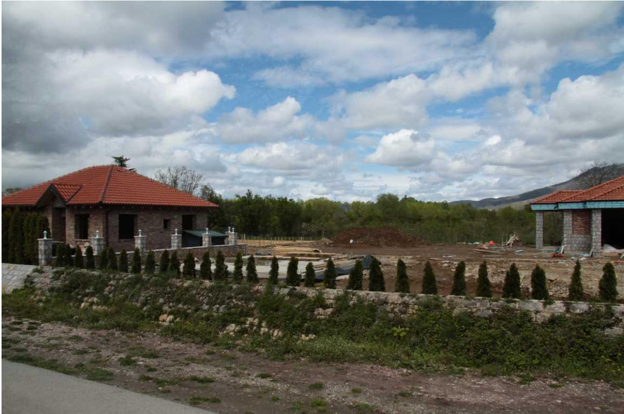
Photo 1: Two new residential buildings under construction on the border with Gorica North area. @A.Sovinc.
