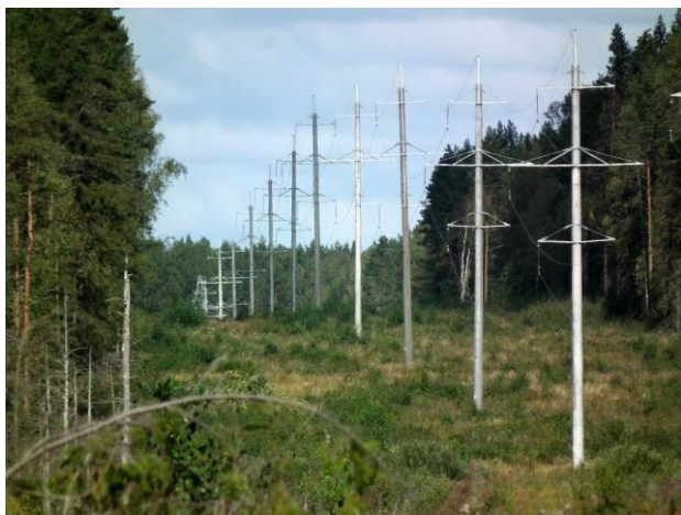
Picture 6. Illustrative picture – a similar 35 kV power line is planned for construction at Olmany
