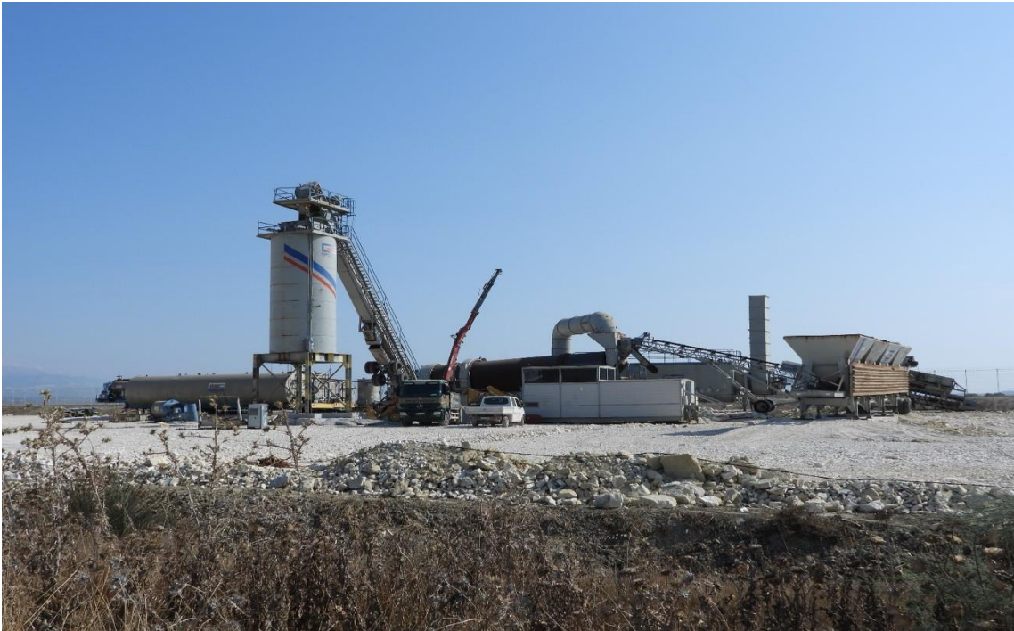
Figure 8: Machinery for the production of concrete or asphalt, newly established outside the fence of the construction site 25.07.2024 © Zydion Vorpsi/PPNEA
