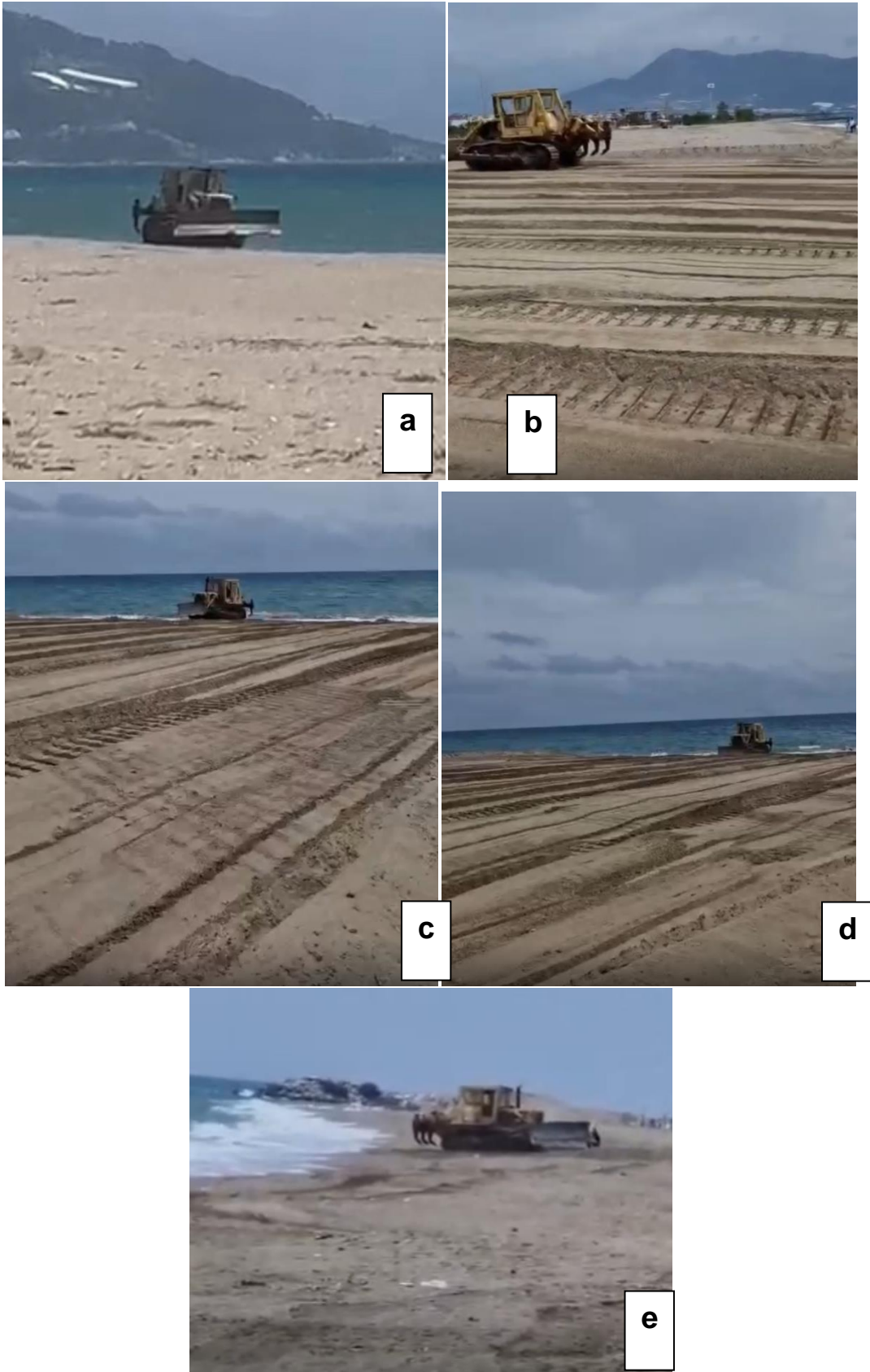
Figure 5 a-e - Plowing of the nesting beach with construction equipment - 20.04.2024
