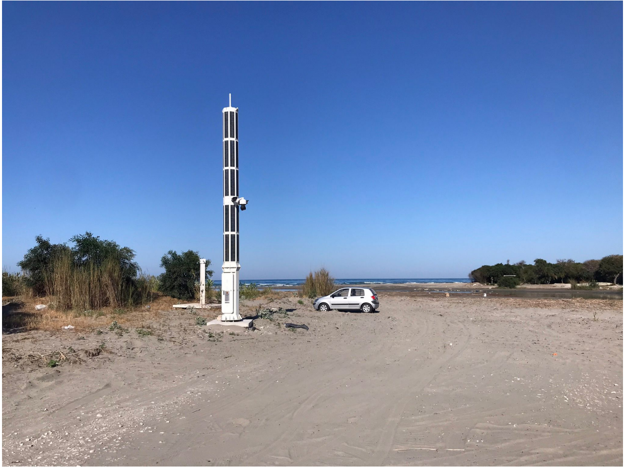
Installed cameras. (Fig. 21)
