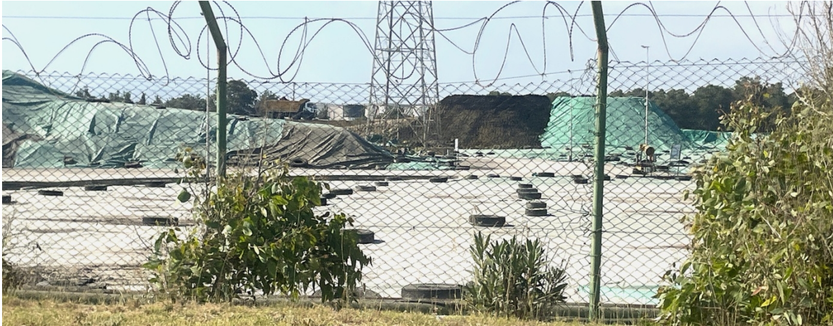
Figure 13. Operations and activities conducted within the chrome waste storage area.
