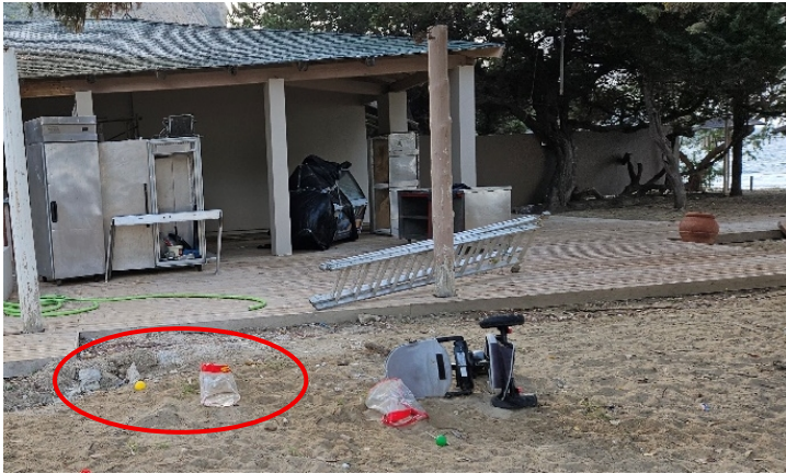
Photo 4c: Expanded wooden decking. Concrete was poured as foundation, indicated by the red circle (Daphni, May 2025).
