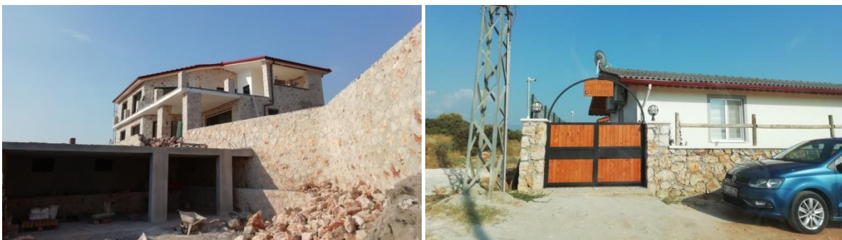
Fig. 42-43. Patara SPA. Construction of 20 additional summer houses that do not seem to have permission.
