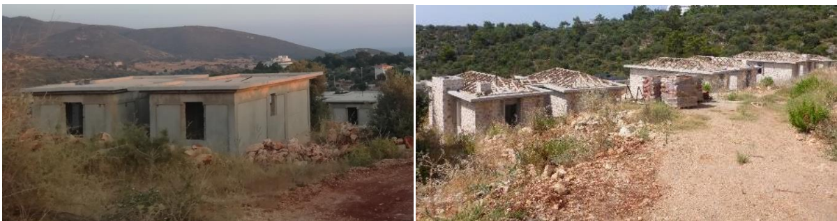
Fig. 40-41. Patara SPA. 3 rd Degree Archaeological Site. Construction work continues for approx. 310 buildings.
