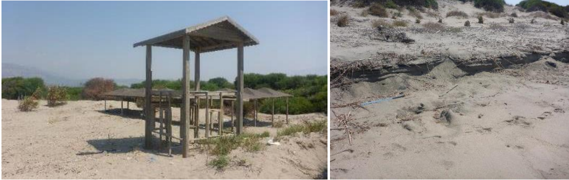
Fig.5-6. Patara SPA. Letoon beach. Left: SPA facilities have been abandoned and have not been removed from the dunes. Right: An old fence line with posts and old wire between dunes and beach.
