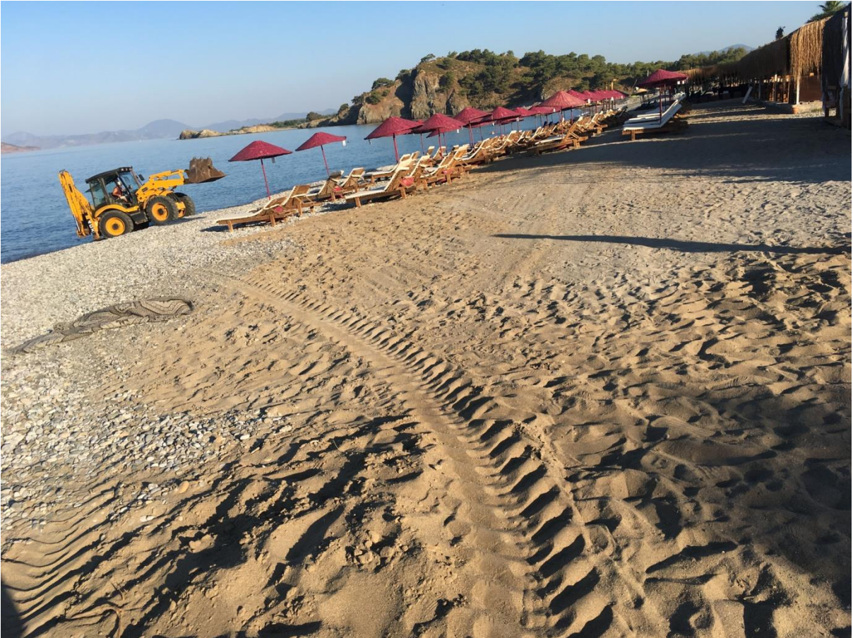
Fig. 37. Fethiye SPA. Çalış. Section B. Sand movement with heavy machinery during nesting season.
