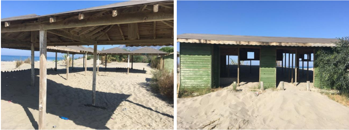
Fig. 4-5. Patara SPA. Letoon beach (north of Esen River outlet). SPA facilities have been abandoned and have not been removed from the dunes.
