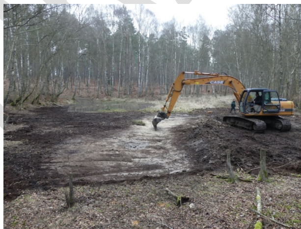
Topsoil and vegetation removal to restore rich acidic forest ponds in Rambouillet forest, France - A. Potier CBNBP/MNHN
