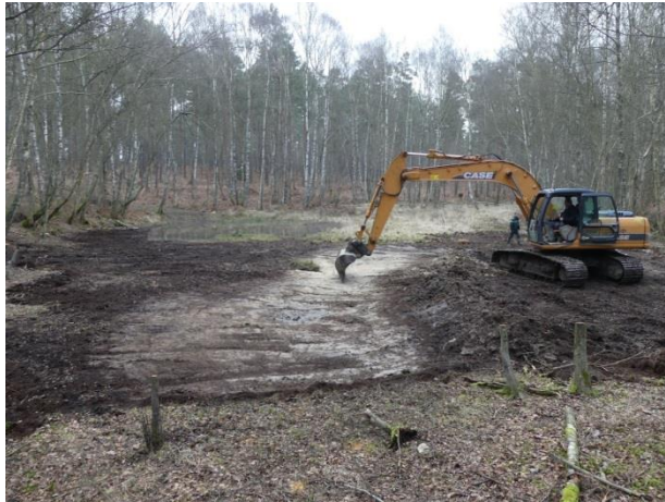
Topsoil and vegetation removal to restore rich acidic forest ponds in Rambouillet forest, France - A. Potier CBNBP/MNHN
