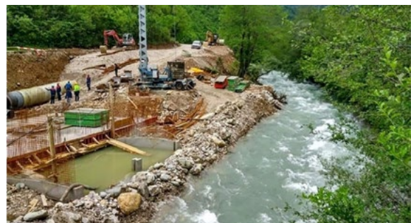
Small hydropower plant "Zlate", river Doljanka, Jablanica, Bosnia and Herzegovina
