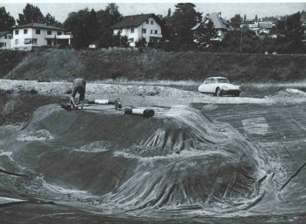
"Wetlands are never wastelands" — Wastelands may become wetlands: an artificial wetland under construction in tiny Liechtenstein which disproportionately contributed to the success of the Council of Europe's wetlands campaign (Photo M. F. Broggi)
