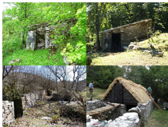
Before and after – Dragodid Association work on restoration of Petrebišća hamlet. © 4 Grada Dragodid
