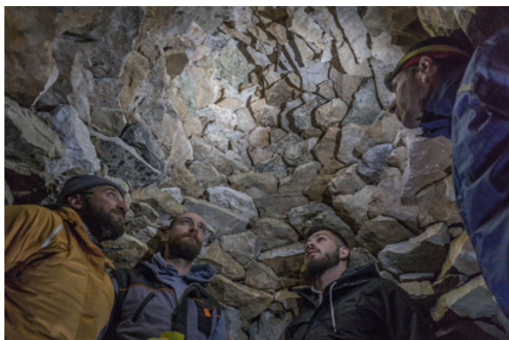
Restoration of kućerica corbelled shelter in Konavli, in collaboration with local stonemasons. © 4 Grada Dragodid
