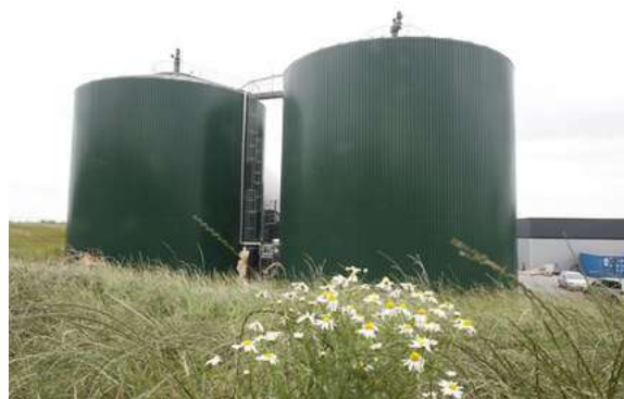
Figure 52. Silos for methane production (Photo: C. Saidou / Ministry of Agriculture, France)
