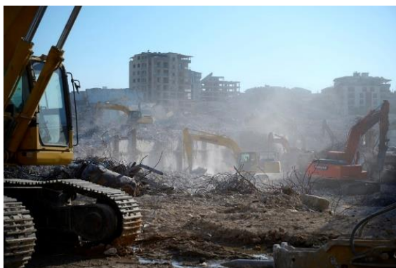
Removing the rubbles in Hatay, Türkiye, in an urban area where search and rescue was not possible anymore
