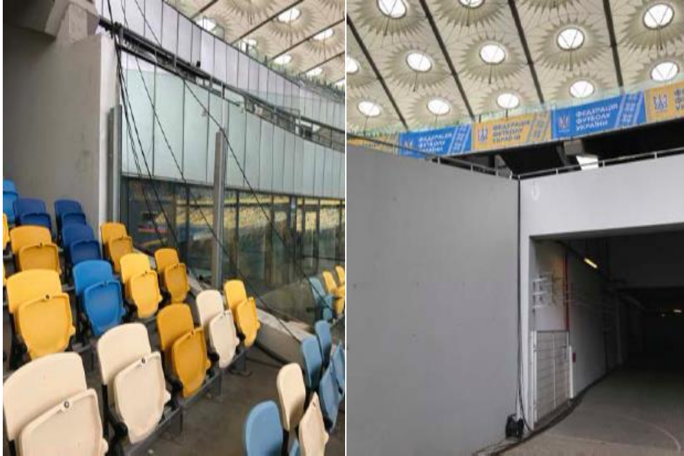
Pictures 22 & 23 –Temporary cabling running through away section
