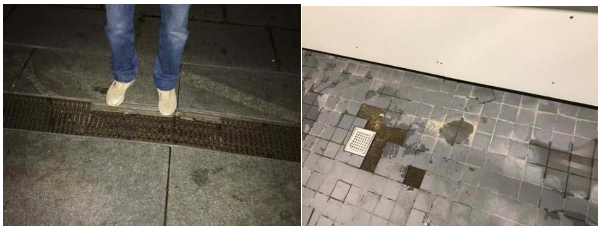
Pictures 16 & 17 – Loose drain covers and tiles
