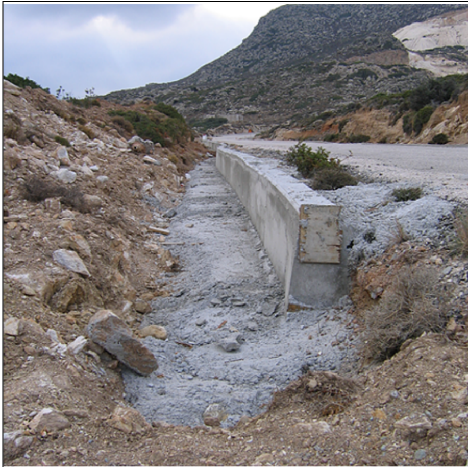
Figure 3-13 Fig. Construction phase of a concrete wall build as an exclusion structure for reptiles on an existing road.
