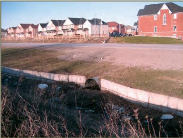
Photo 41. Concrete wall in Aurora, Ontario © K. Gunson
