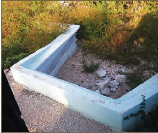
Photo 11. Tunnel with headwalls connected to concrete guide fencing in Cuba. © G. Barrett
