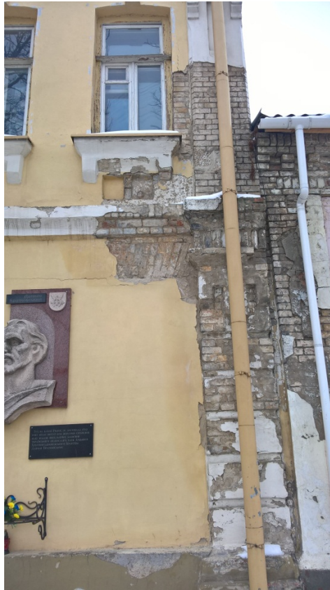
The condition of the building's façade, February 15 th 2017
