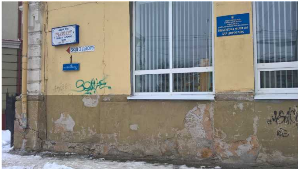
The photo of the neglected house facade. February 15, 2017
