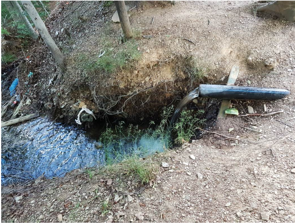
HPP on Belichica River, NP Mavrovo, water discharged inappropriately
