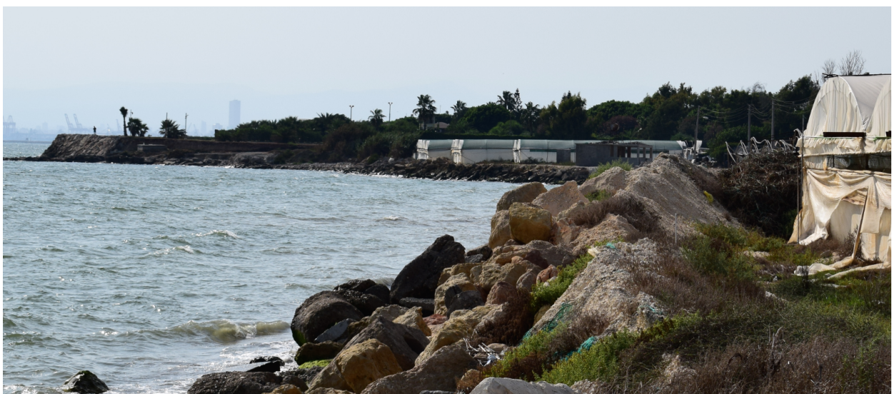
Figure 24: use of rocks and concrete boxes to halt and control the erosion of the coastline
