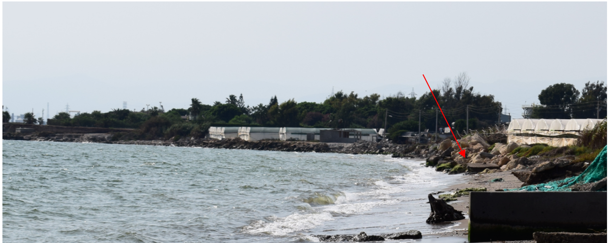
Figure 23: Coastal erosion in K3 area; use of rocks and concrete boxes to halt and control the erosion of the coastline
