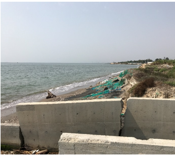
Figure 20: effects of coastal erosion
