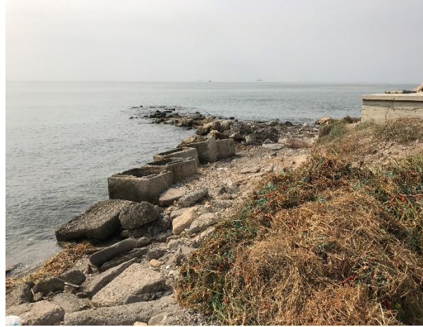
Figure 19: use of rocks and concrete boxes to halt and control the erosion of the coastline
