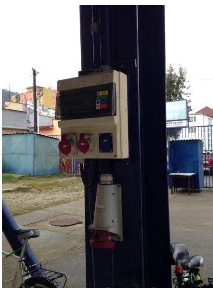
Unprotected electrical apparatus
