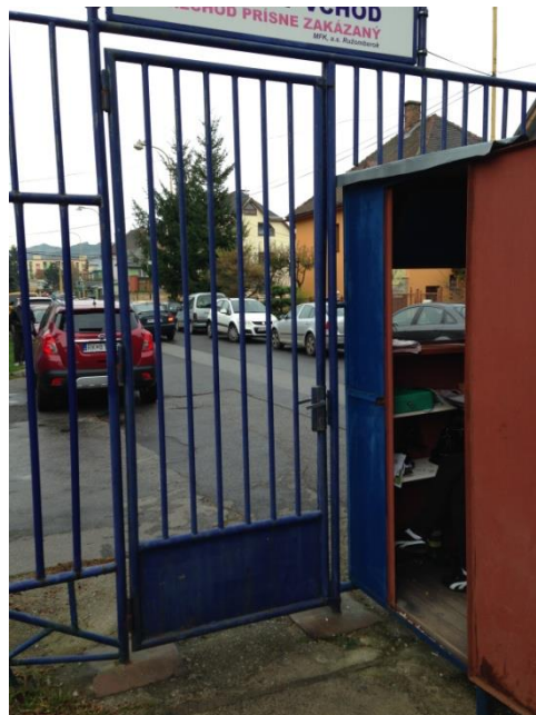
Entry system for fans via steel gate
