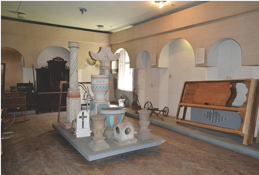
The interior of the Gendler House: illustration of inadequate construction and installations
