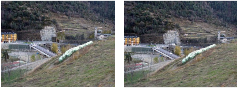
Figure 14: North entrance, initial stage on the left and final stage on the right
