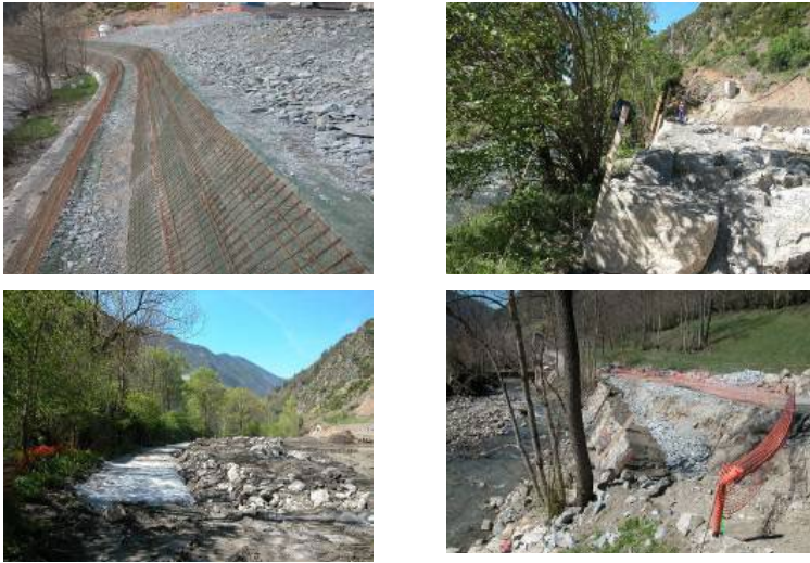
Figure 22: Top left-hand photograph: reinforced earth wall; other photographs: stone wall.
